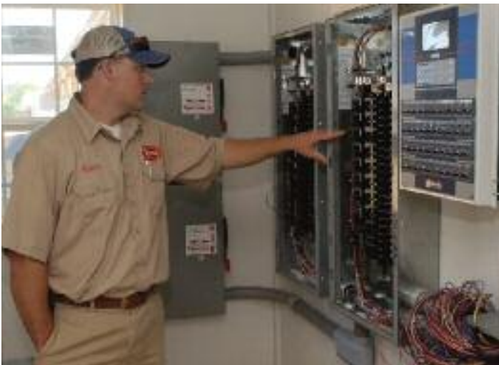
Inspecting new construction is part of the job. Here he checks the control room wiring in a new 66 x 500 ft. house owned by Tyson Blountsville live haul supervisor Andy Graveman.
